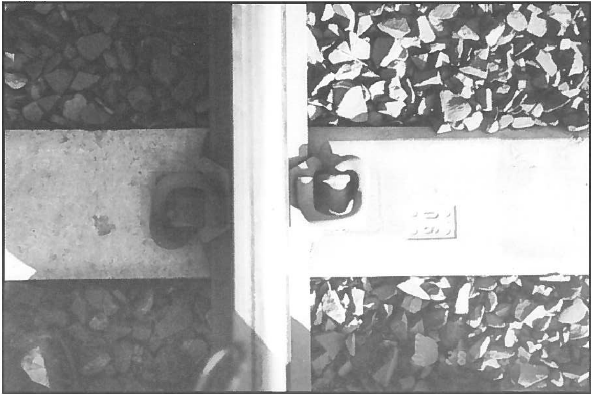
Photo 12: Concrete tie - Pandrol e-clip
