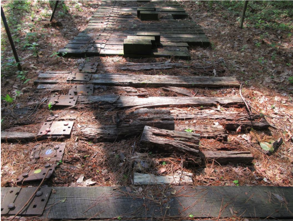
Figure 2 – Control ties showing signs of severe deterioration
